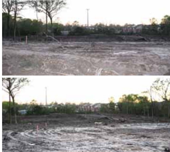
Figure 7: Typical Development, no erosion control measures employed
