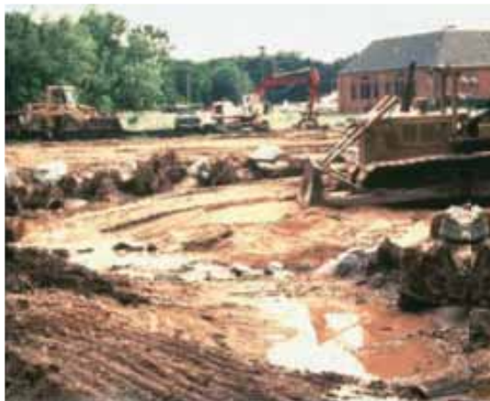
▲ Figure 24: Construction activities in violation of the Water Quality Act
